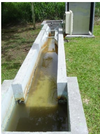
Figure 2.4 – Canal venturi sortie station
